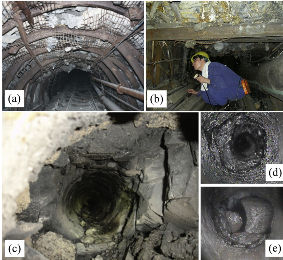
Fig. 2. Deformation–failure of roadway and horizontal borehole in underground coal mine (Luo et al., 2010; Zhang et al., 2009).
