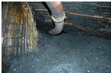
图 1 海孜煤矿 1026 机巷掘进工作面突出情况 Fig.1 The outburst situation of the II1026 heading face in the Haizi Coal Mine
